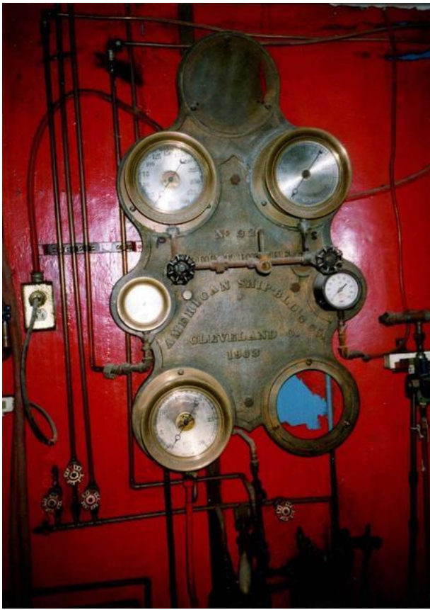
Above: Gauge board on J.B. Ford's triple expansion steam engine. John Belliveau photo
